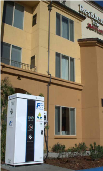
Fuji DC Fast Charger at the Residence Inn, a Marriott Hotel in San Juan Capistrano, CA.
